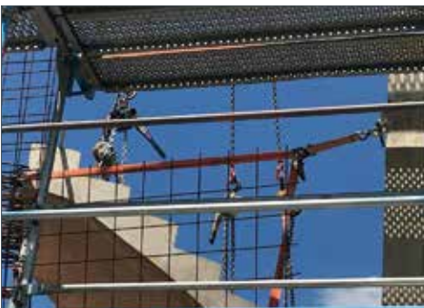
Positioning work with dynamic loads Especially when using multi-fall chain slings (e.g. installation of turbines)
